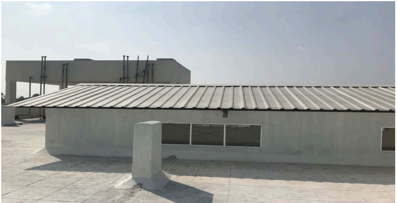
Meta color sheet roofing over the skylight on Hostel Block II. In the background is overhead tank.
