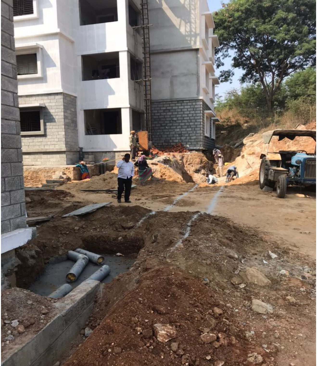
Front road adjacent to the entrance gate and overall drainage system of the Hostel Blocks under progress
