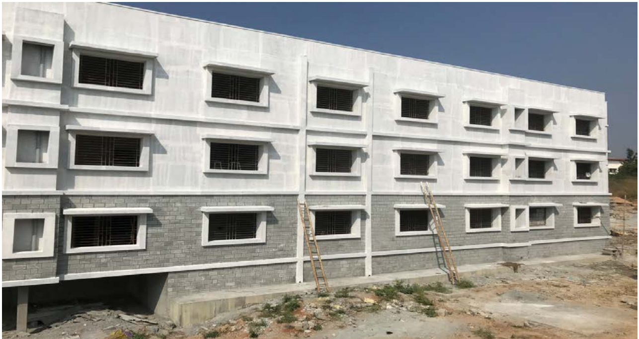
Primer painting being done on the eastern part of the building. Site development will follow soon. (BOY'S HOSTEL II)
