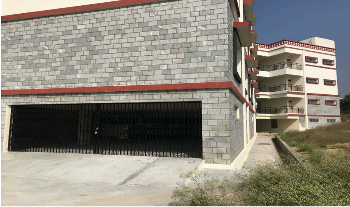
Drainage work and basement with shutter being used as a garage - completed
